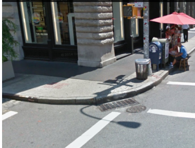
No Curb Ramps
